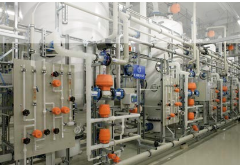
Ultrapure water generation system
